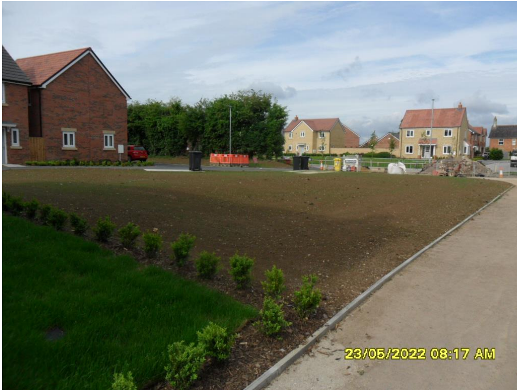
9-Straps not nailed to rails, nail as necessary, pic below.
