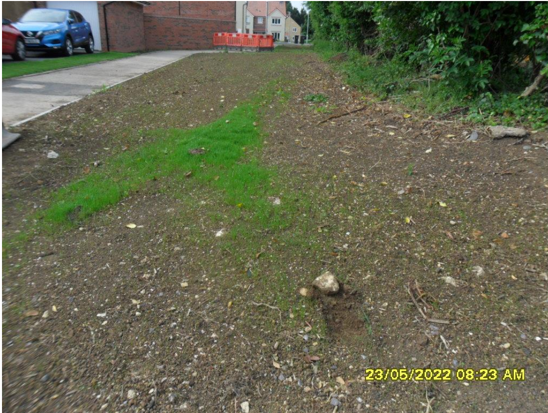
24-level up with top soil and apply grass seed to take out trip hazard between open space and kerb as necessary across open space pic below.
