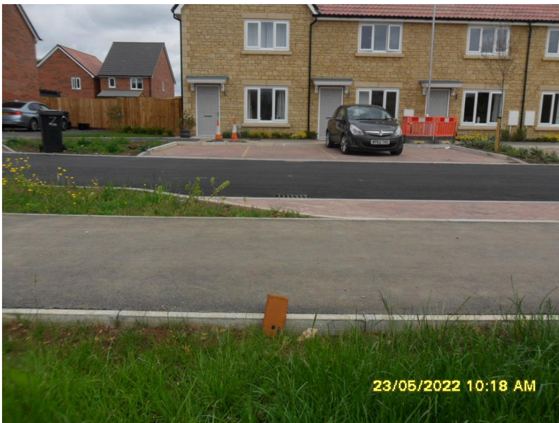
25-Foot path not installed, gravel with timber edging as per spec, pic below.
